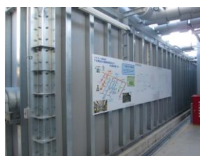
Fig.2 Ice storage tank
